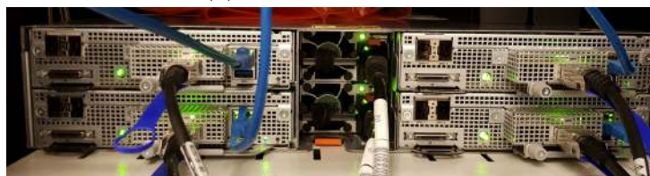
(b) Back of the servers
