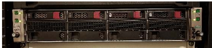
(a) Front of the servers
